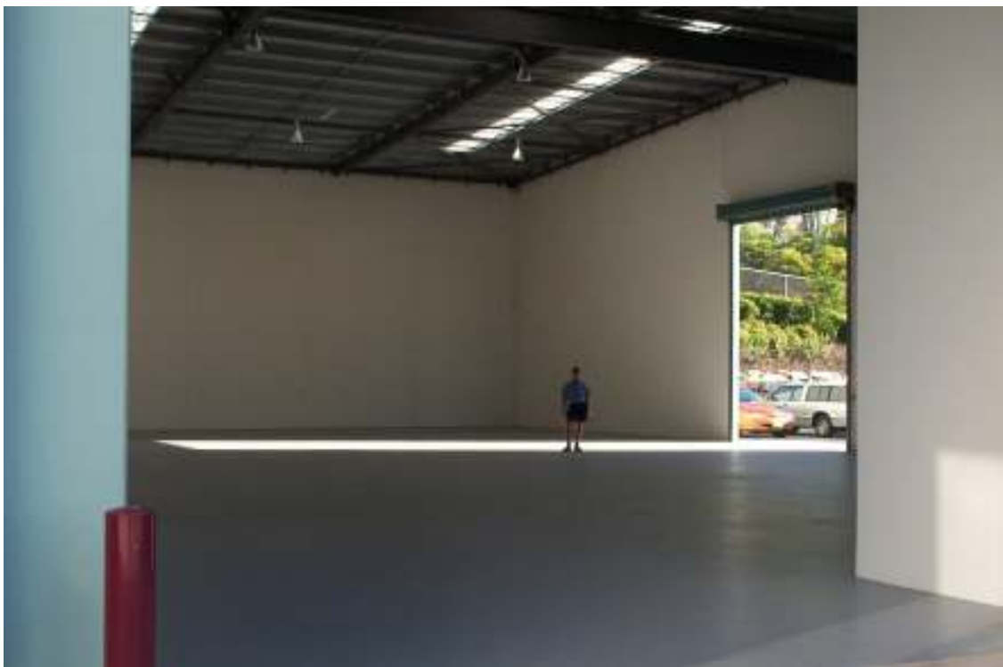
Warehouse – To be repainted prior to Occupation
